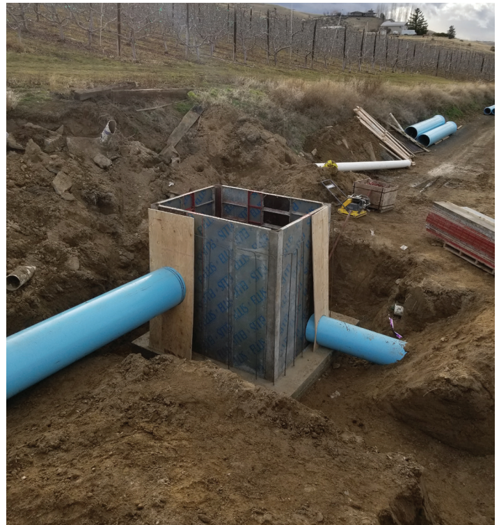
The piping of the lower sections of the Selah-Moxee Canal in Moxee, Washington.
